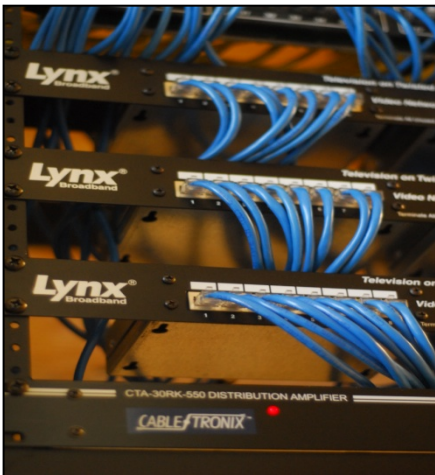
Wiring closet at the hotel
